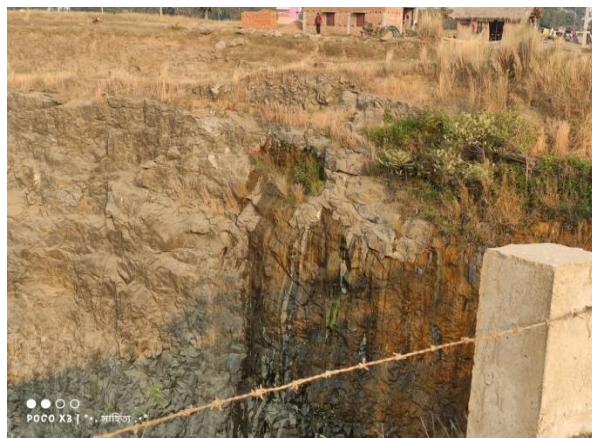
Water seepage through underneath rocks
