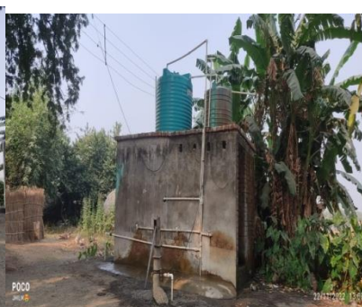
Hand Pump & Sanitary toilet
