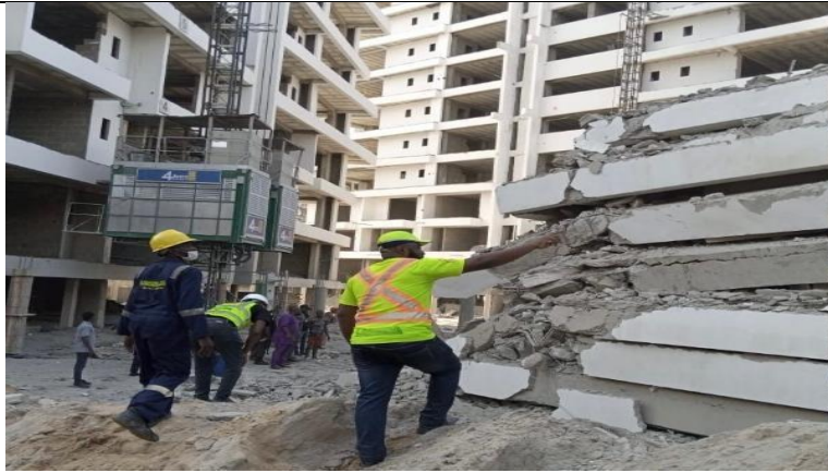
Figure 1: 21-A building collapsed on Gerard Road, in the highbrow area of Ikoyi, Lagos
