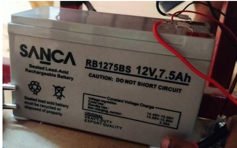
Fig5.4: Rechargeable lead-Acid Battery
