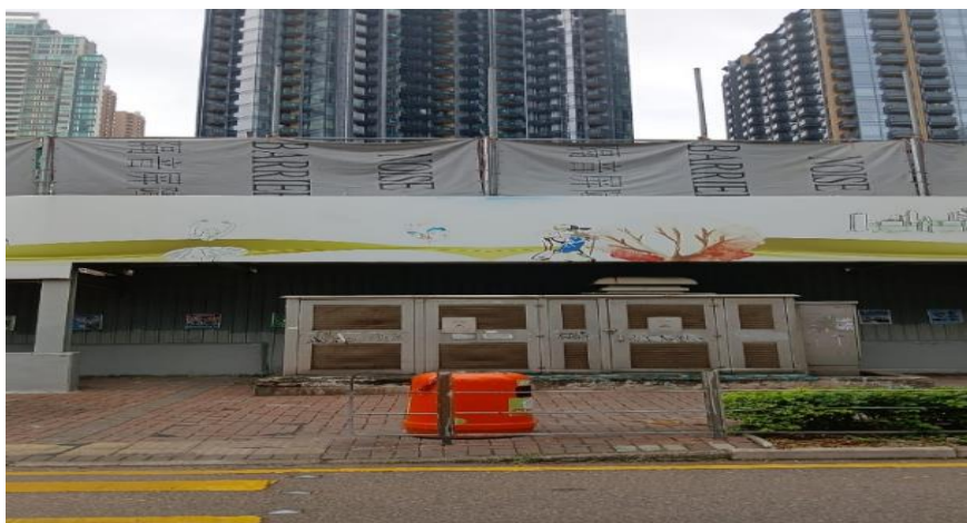
Figure 1: Typical temporary outdoor transformer room
