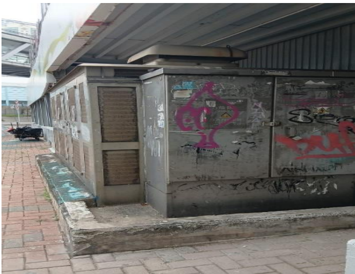
Figure 3: Control panel is mounted outside of transformer room
