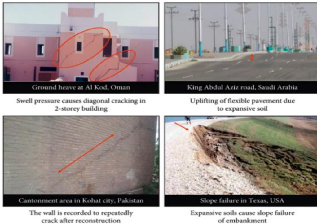
Figure 1: Expansive soil damage to civil engineering infrastructure across Oman, KSA, Pakistan, and USA (with some changes for comparison purpose) (43)
