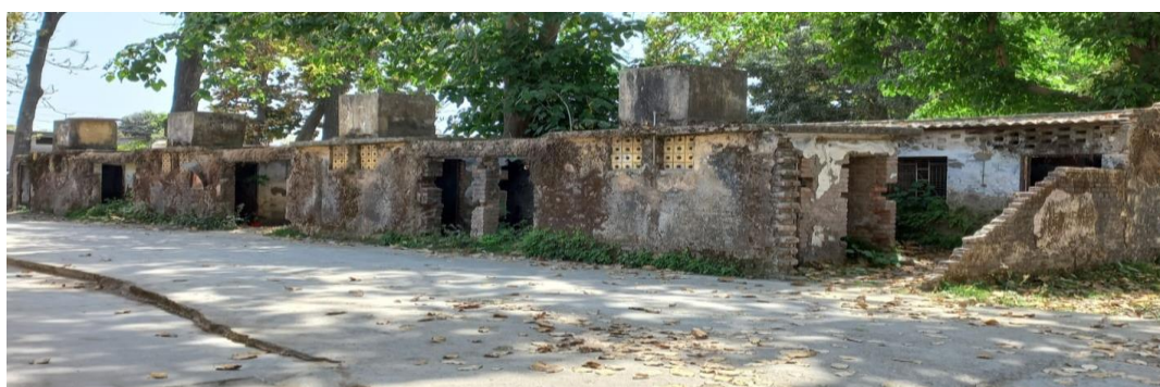
Figure. 1.a: Building in dilapidated condition near Aadarsh Colony
