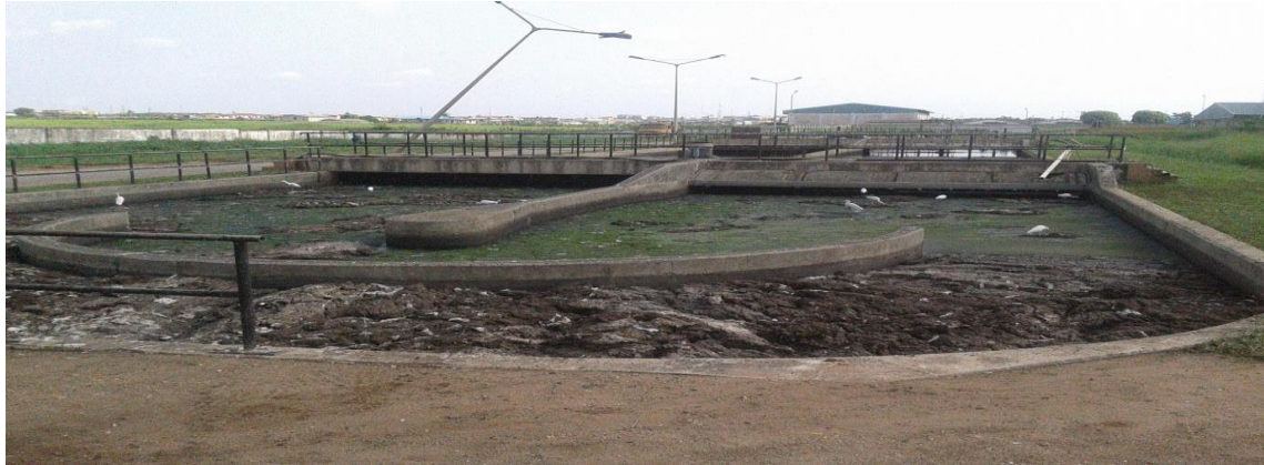
Plate 3.1. Field survey photograph of the unserviceable sewage treatment plant equipment at MMIA.
