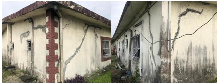
Fig.(2) Differential settlement evidenced by cracks on the building
