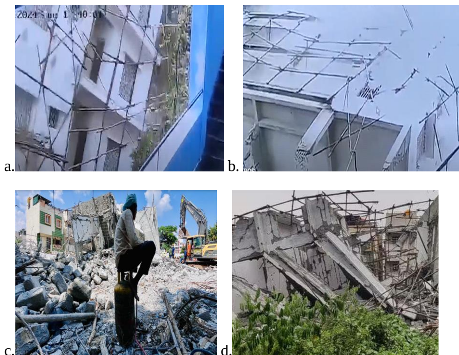
Fig 4: (a and b): The dilapidated building (The India Today), (c) The demolished building (The Hindu): (d) The structural failure from Back (The Mint)
