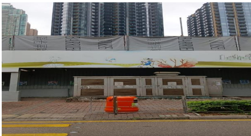
Figure 1: Typical temporary outdoor transformer room
